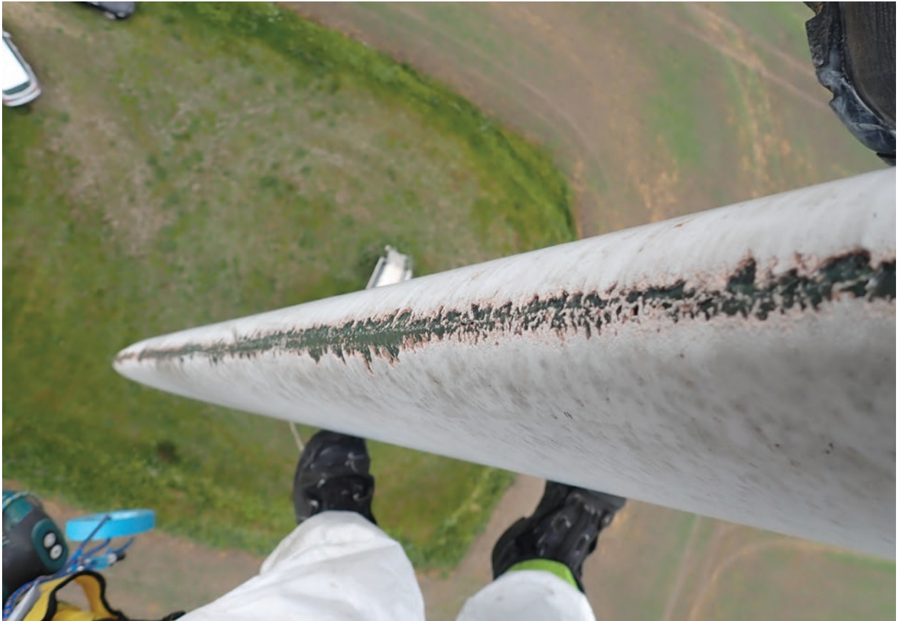
Figure 3: Damaged wind-turbine leading edge. (Courtesy: Belzona)
