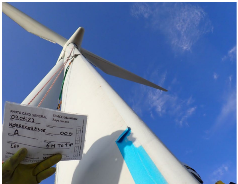
Figure 1: Leading edge protection of wind turbine blade using polymeric technology. (Courtesy: Belzona).
