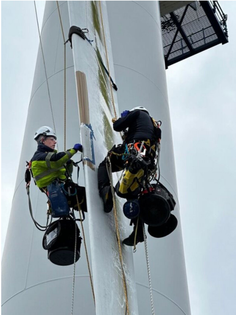
Technicians Warren Mills (left) and Jean Pieree Alcantara (right) complete GEV's new blade repair training course at Port of Blyth's Port Training Services turbine facility. (Courtesy: GEV Wind Power)
