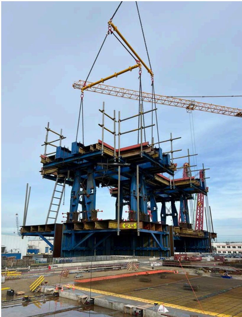
Construction on the Princess Elisabeth island will run until the end of 2026. (Courtesy: Modulift)
