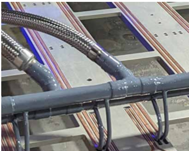
Heresite™ coated copper tubing and stainless over-braid flex lines. (Courtesy: ACT)
