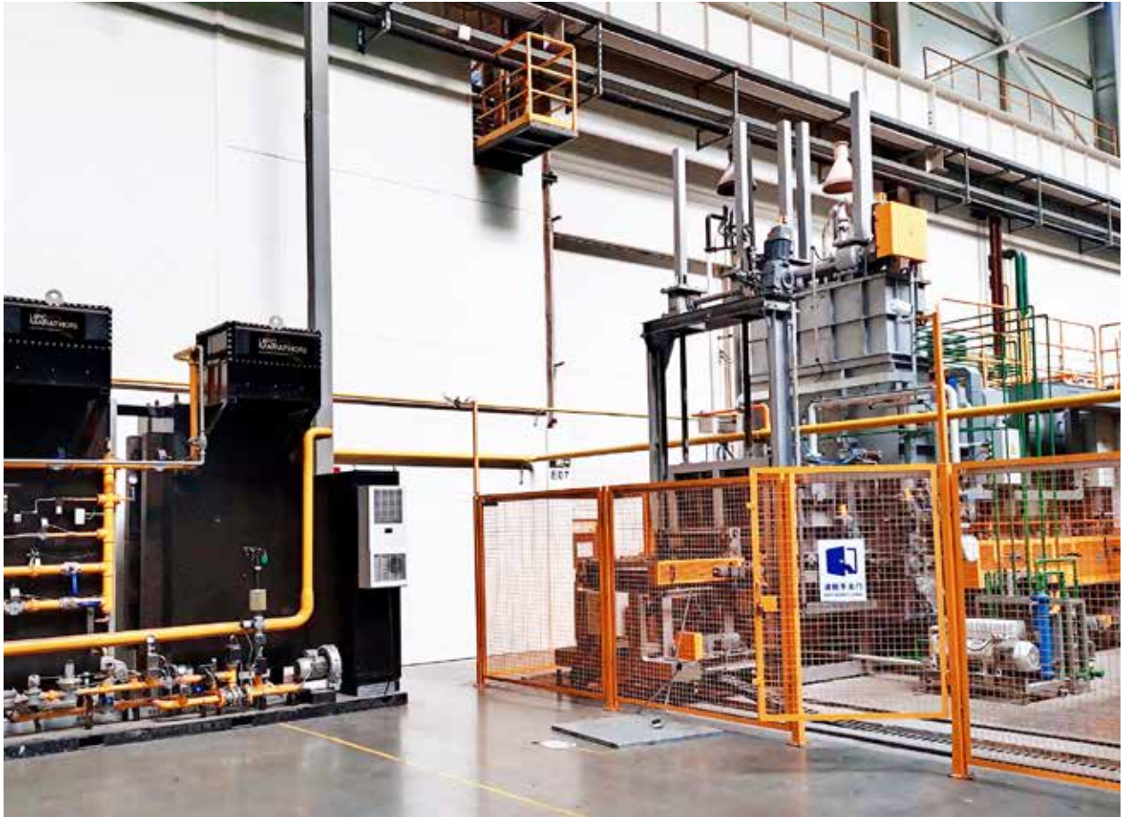
NGC Gears has integrated two more EndoFlex endothermic gas generators into its China facility. (Courtesy: NGC Gears)
