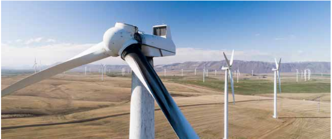
Figure 2: Blade failure at a U.S. wind farm. (Courtesy: The Oregonian, 2022)
