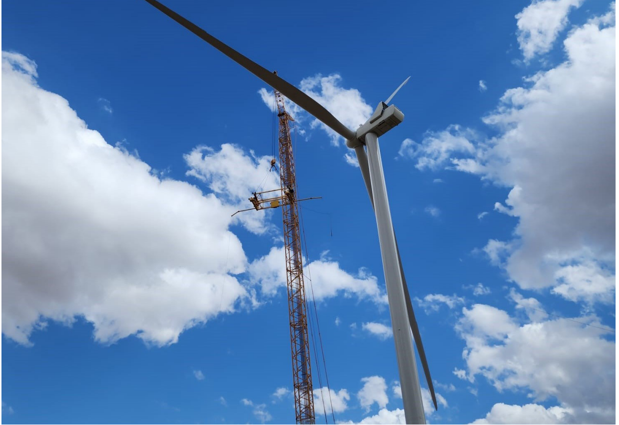
The Whitla Wind facility has an installed capacity of 352.8 MW, which allows it to generate enough energy to power more than 100,000 homes per year. (Courtesy: Sarens)
