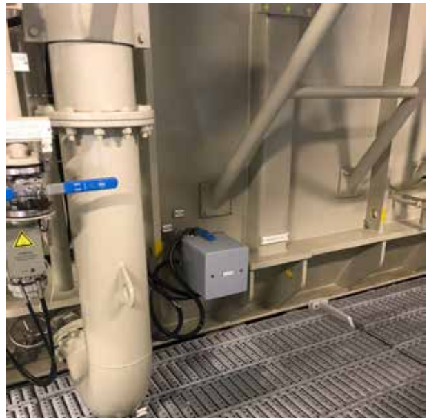
An on-line DGA system installed at Hornsea II offshore wind. (Courtesy: ZTZ Services International)
