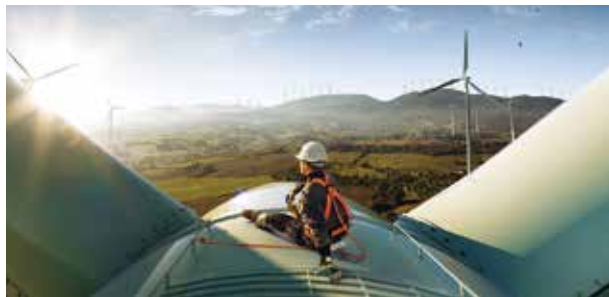
Emerson installs enhanced control strategies and software that optimize wind-turbine and wind-farm output to provide the lowest cost of energy. (Courtesy: Emerson)
