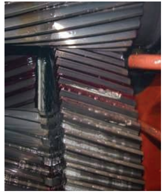
Fig. 2: A damaged gearbox is pictured here.
