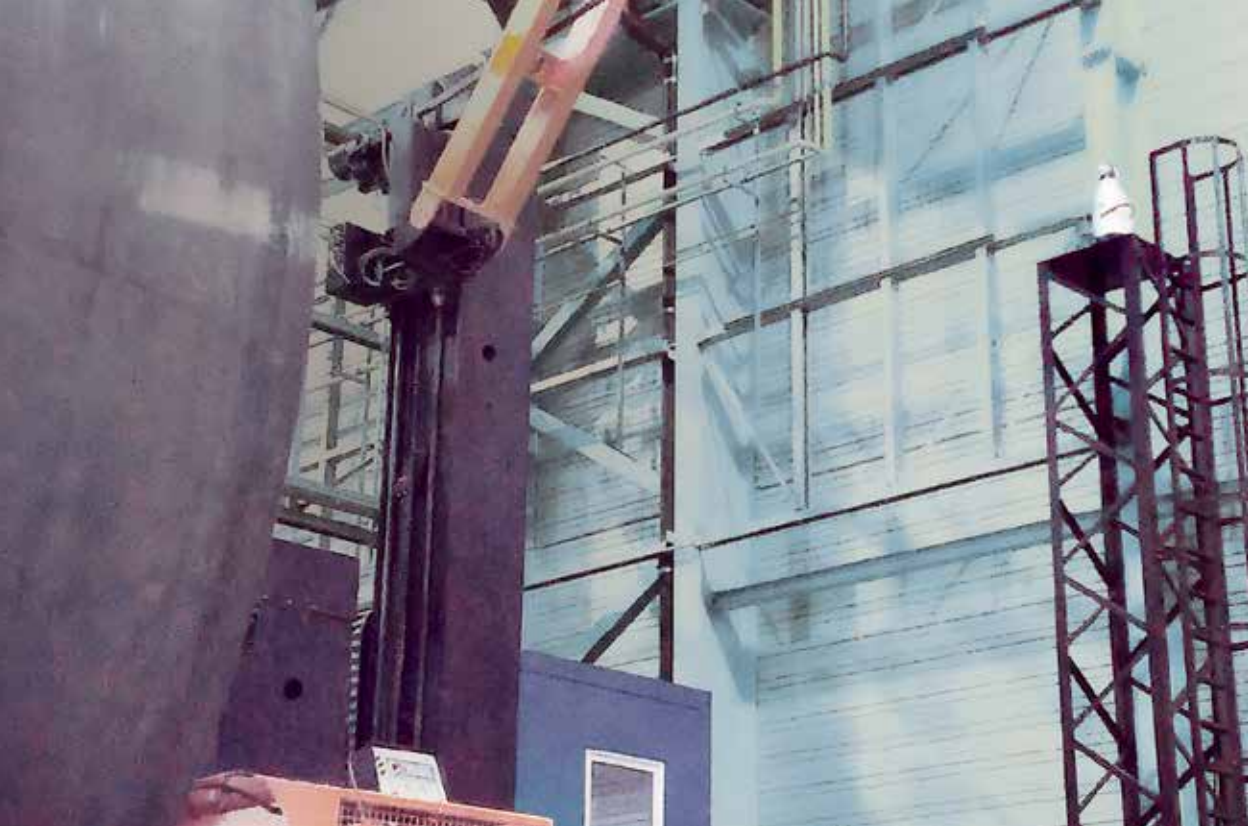
Fig 3: The Leica Absolute Tracker (upper right) is positioned to measure the top of the oversized tubes.
