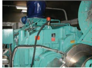
Fig. 2: An oil inlet on top of the gearbox for the return hose from the filtration unit.
