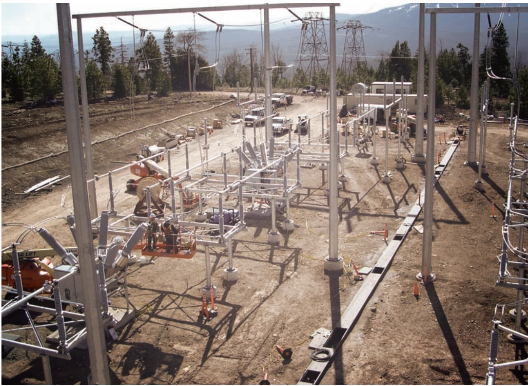
Fig. 4: The Carberry switchyard in springtime.
