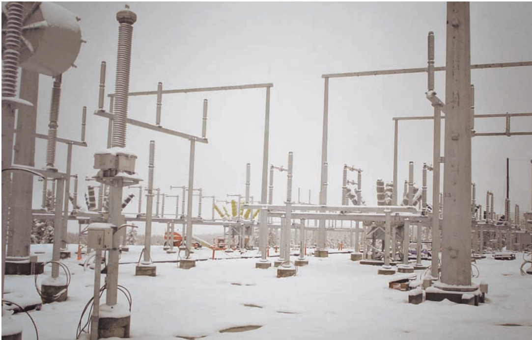
Fig. 5: A shot of the Carberry switchyard under snow in deep winter.
