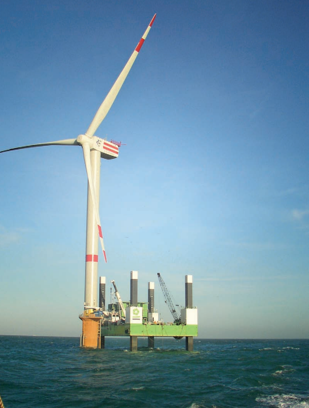
Fig. 3: Isolated tower platforms must be able to provide months of unattended, maintenance-free operation.
