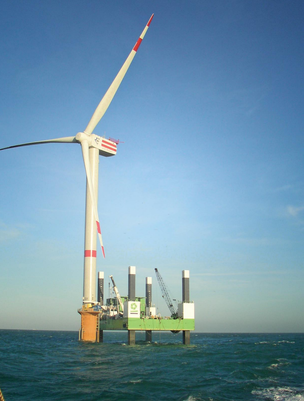
Fig. 3: Isolated tower platforms must be able to provide months of unattended, maintenance-free operation.
