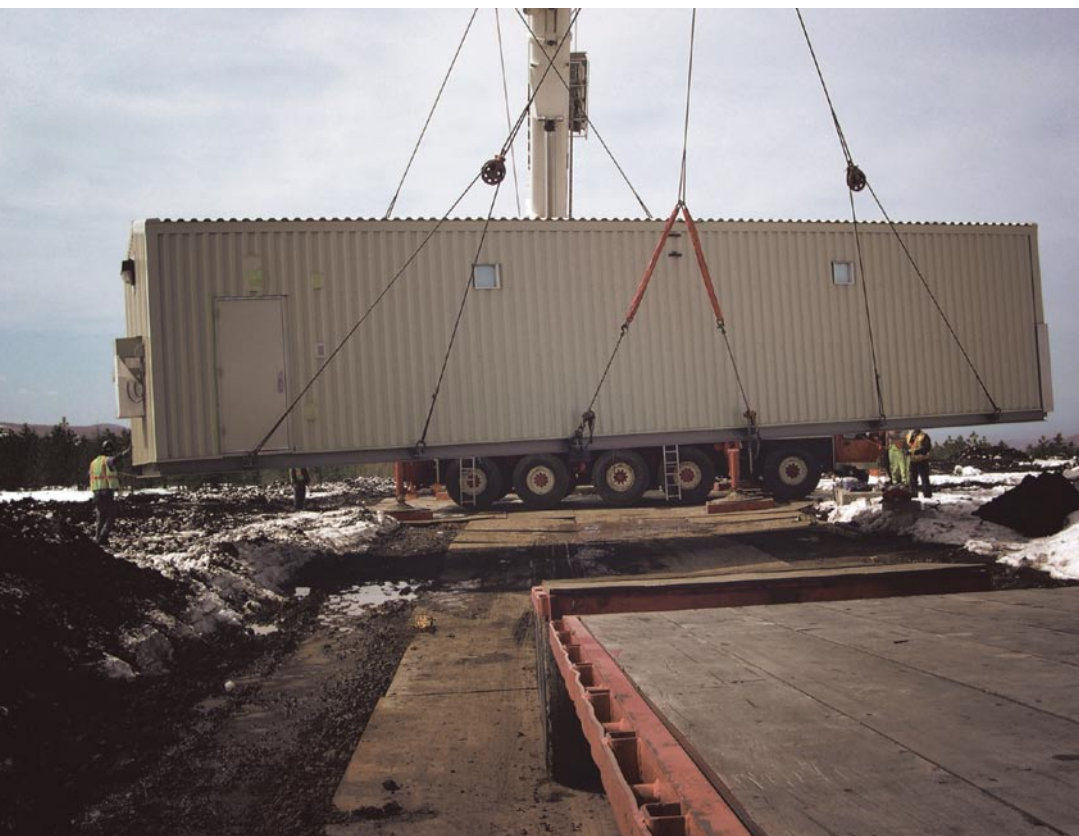
Fig. 3: The control building is mounted at Hatchet Ridge.
