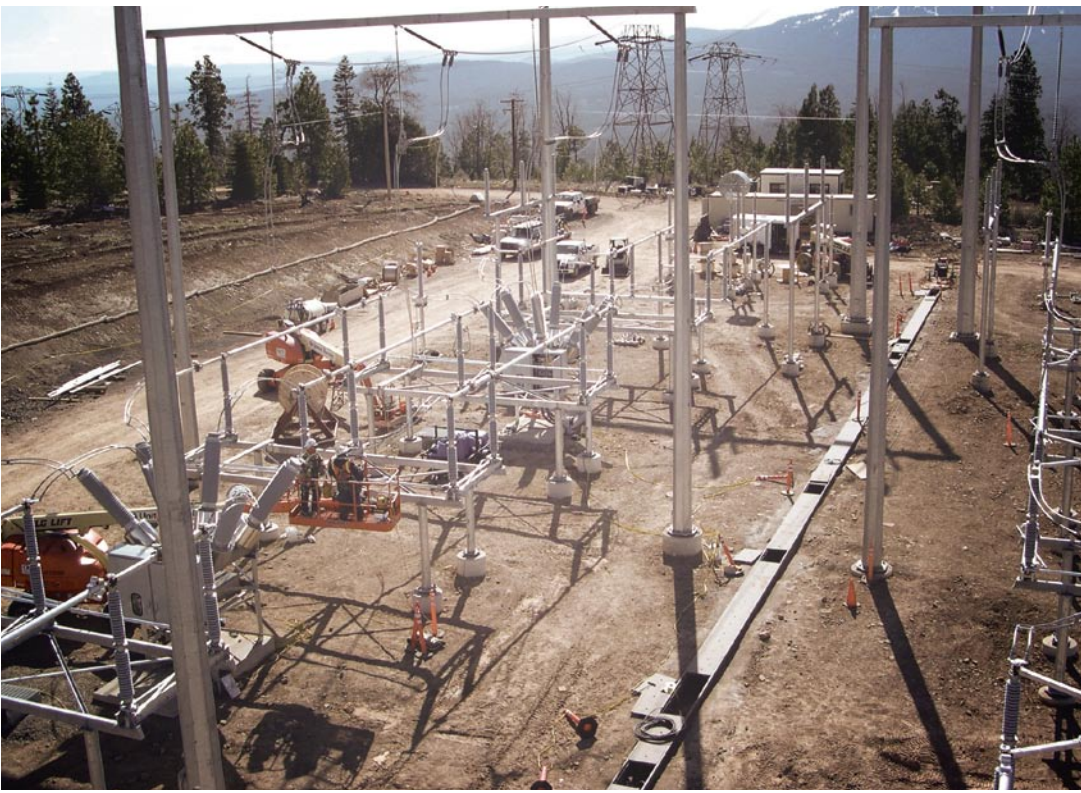
Fig. 4: The Carberry switchyard in springtime.
