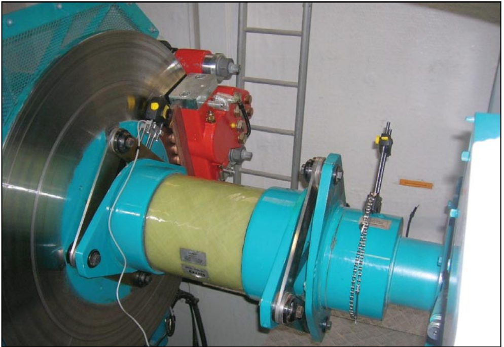
Fig. 5: A laser emitter is mounted on a magnetic bracket with offset adapters directly to the brake disc on a Suzlon gearbox output shaft (Jack Jackson, Alignment & Condition Monitoring, Inc.)
